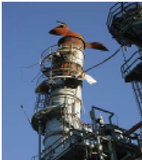
This accident investigated by and picture provided by the U.S. Chemical Safety and Hazard Investigation Board. Visit their site at http://www.csb.gov
